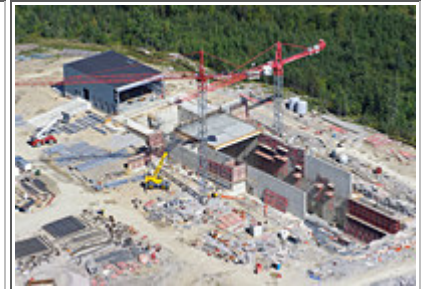
Far detector site is under construction in northern Minnesota. (click for high-res version)
