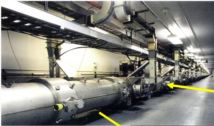
Cryomodules in the accelerator tunnel
